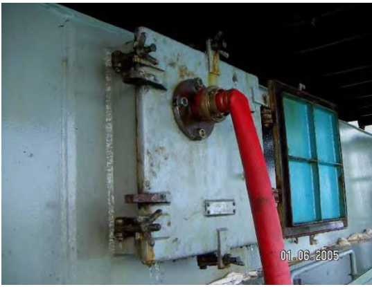
Figure 24, Modified ventilation flap on the CMS PUNJAB SENATOR Source: (Bundesstelle für Seeunfalluntersuchung, 2006, p. 9 Reederei Laeisz)
