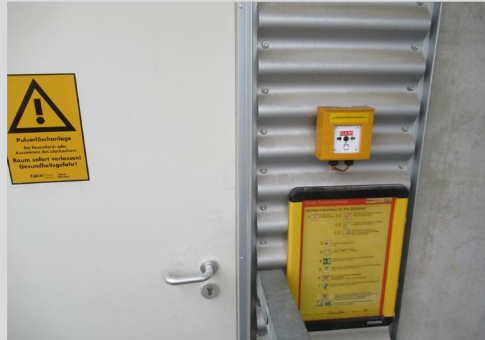
Photo 2: Switch next to mandoor
