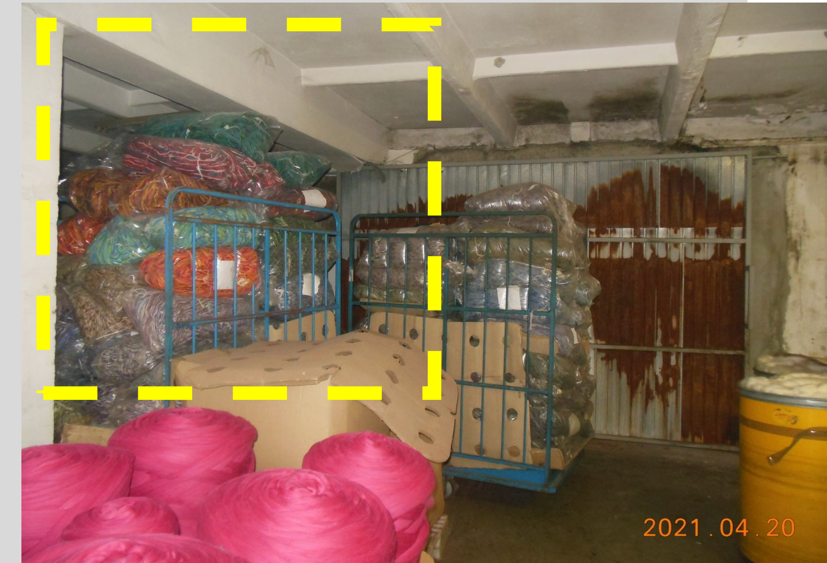
Photo 3: Fire loads up to the roof (heat accumulation)
