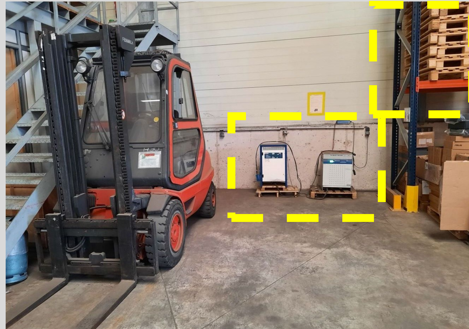
Photo 2: Wooden pallets under charging stations and empty pallets (avoidable)
