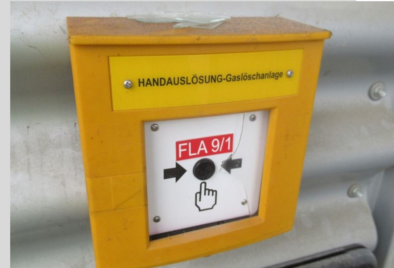
Photo 3: Gas extinguishing system
