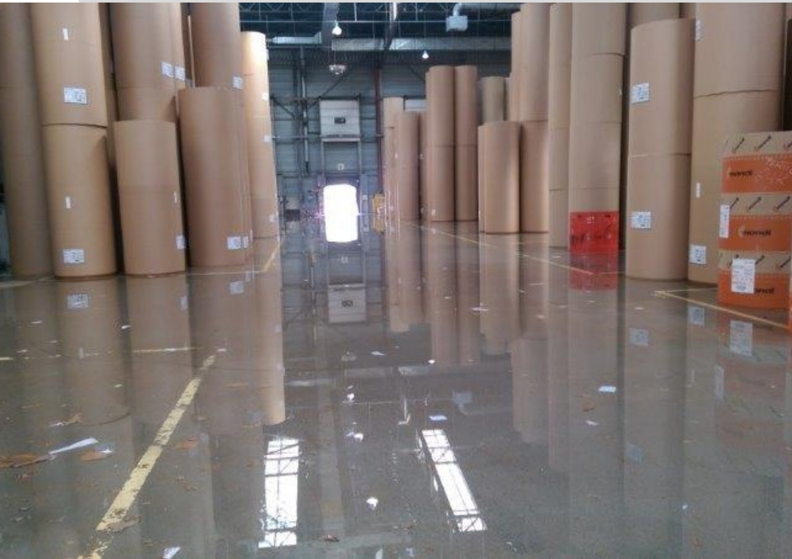
Photo 1: Rainwater in a warehouse with paper reels
