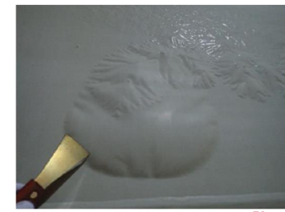
Blistering/delamination due to stress fatigue
