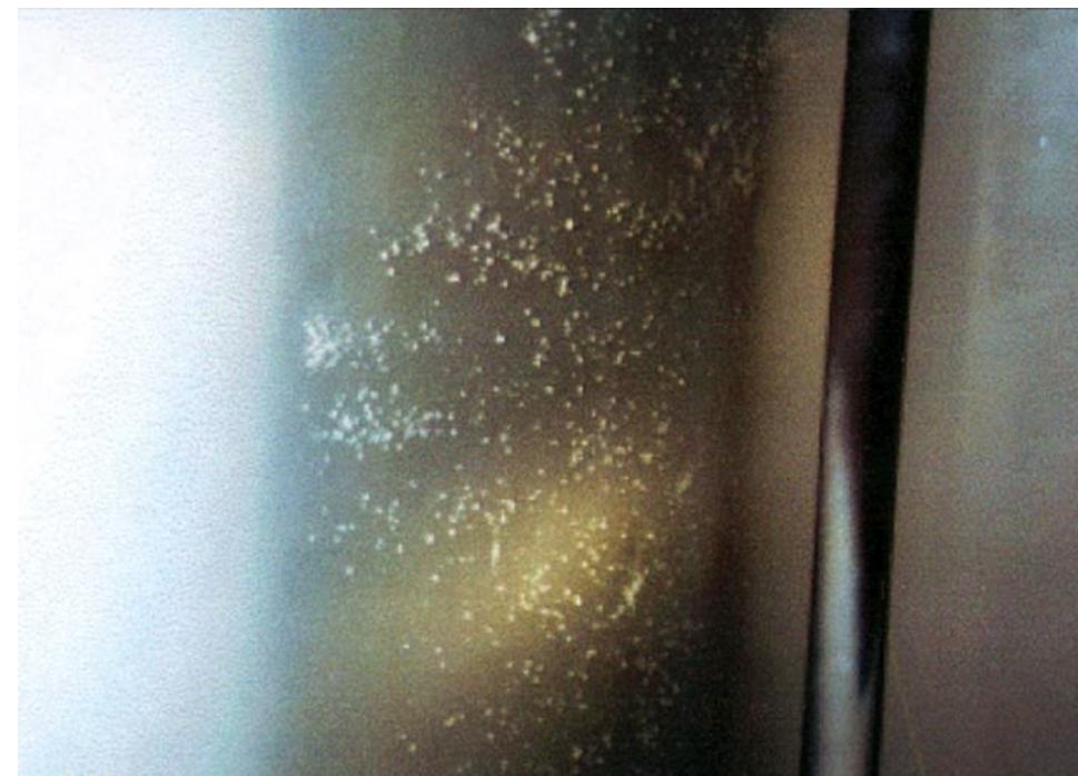
Dryspray not removed
