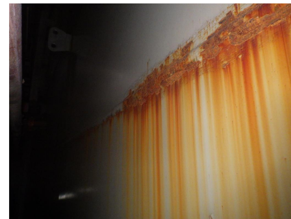
Macrocracking and corrosion on welds for LA coatings
