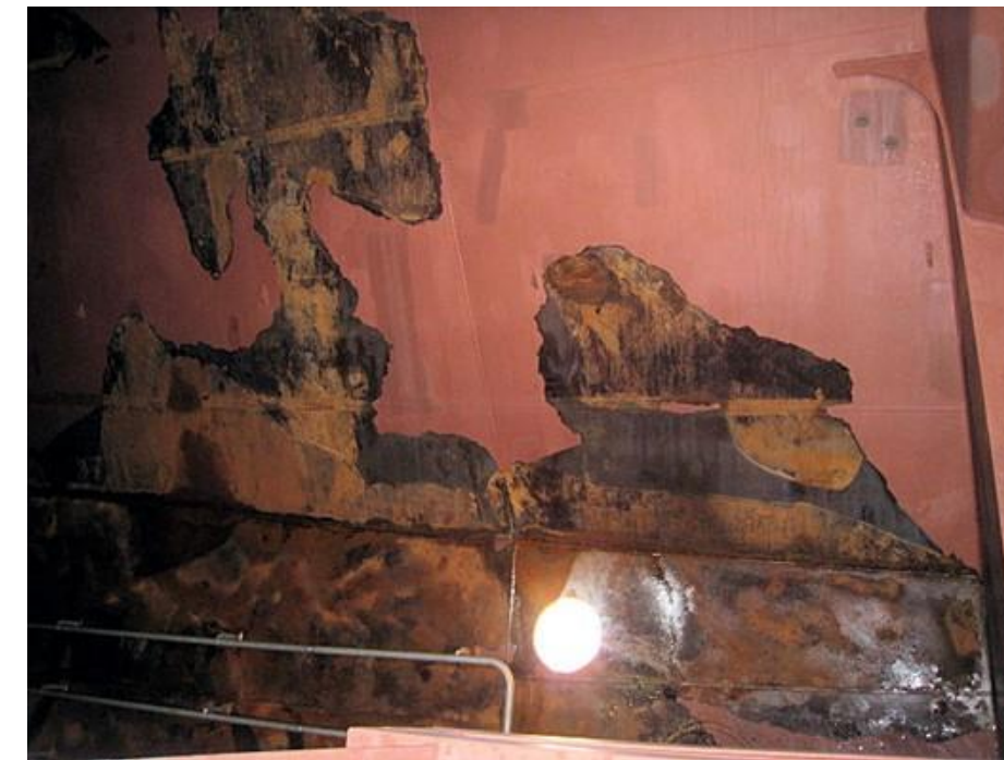
Corrosion/flaking due to insufficient resistance
