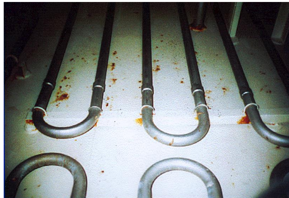
Corrosion due to incomplete cleaning before application
