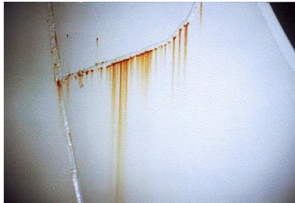
Corrosion due to incomplete stripe coating
