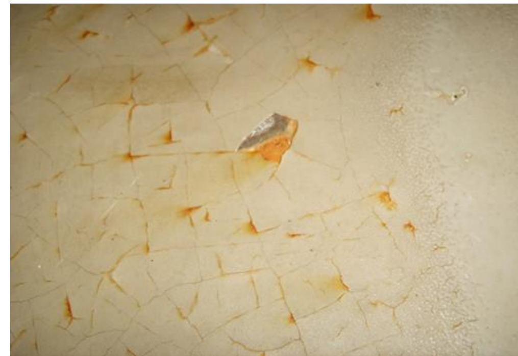
Cracks due to too high DFT or solvent retention
