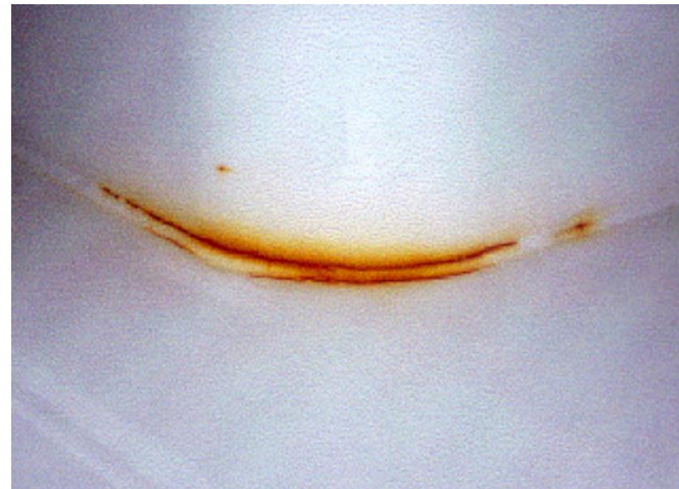
Cracking due to too high DFT & stress
