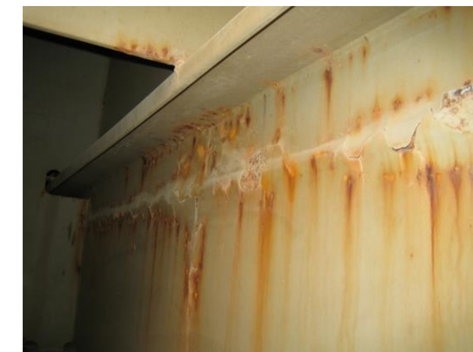
Corrosion due to lacking stripecoat on welds/edges
