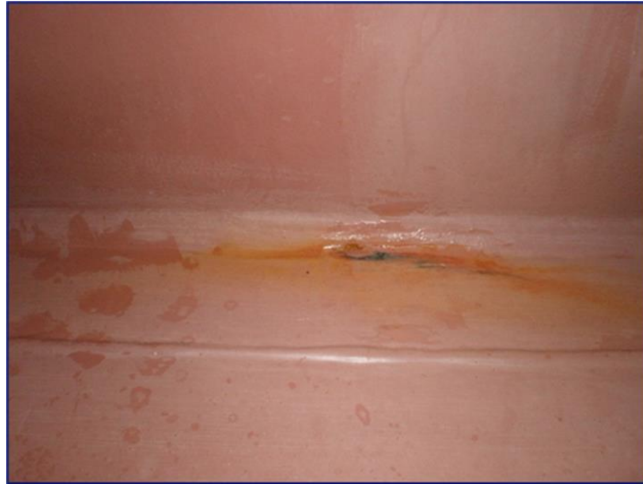
Corrosion due to insufficient steel preparation, P3
