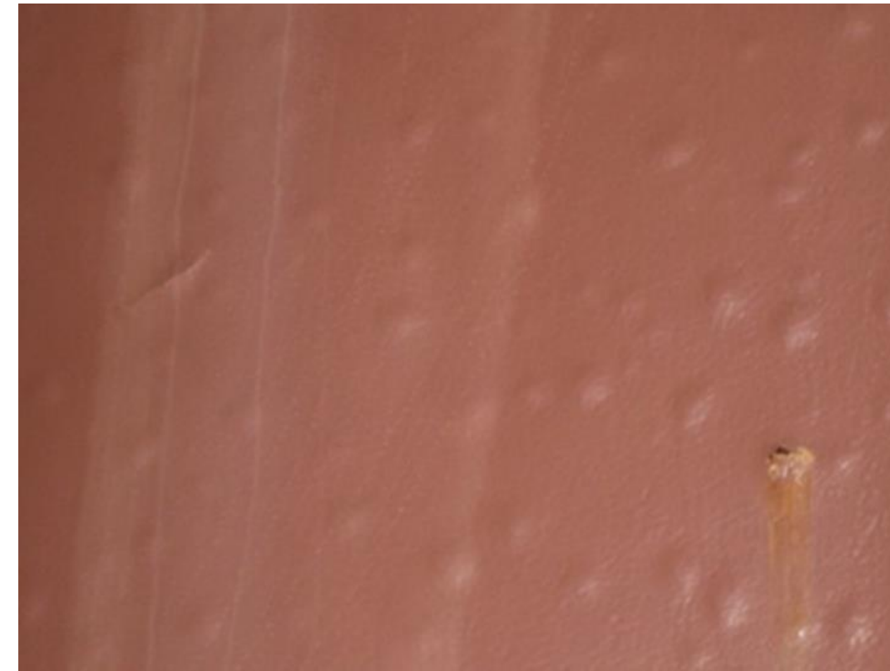
Blistering due to soluble salts on surface
