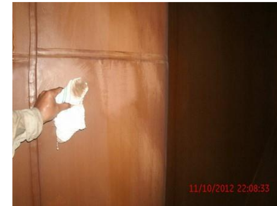
Surface contamination due to insufficient cleaning
