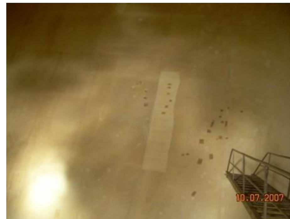
Mechanical damage from dropping tools from ladder
