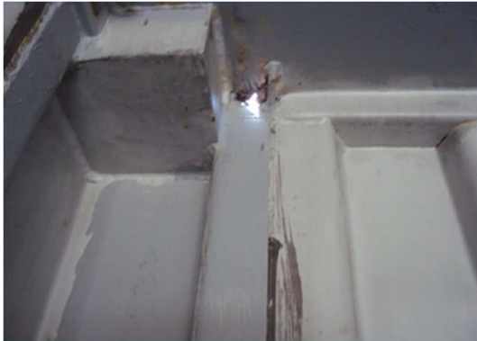
Holes in the container
